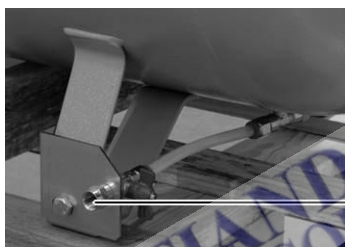
Condensate drain valve on air receiver
