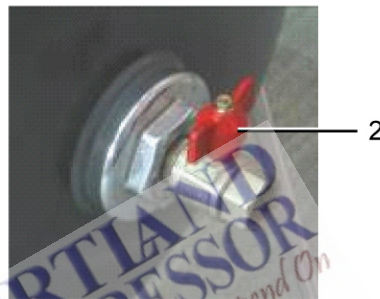
Figure 40: Air outlet valve on the air receiver
